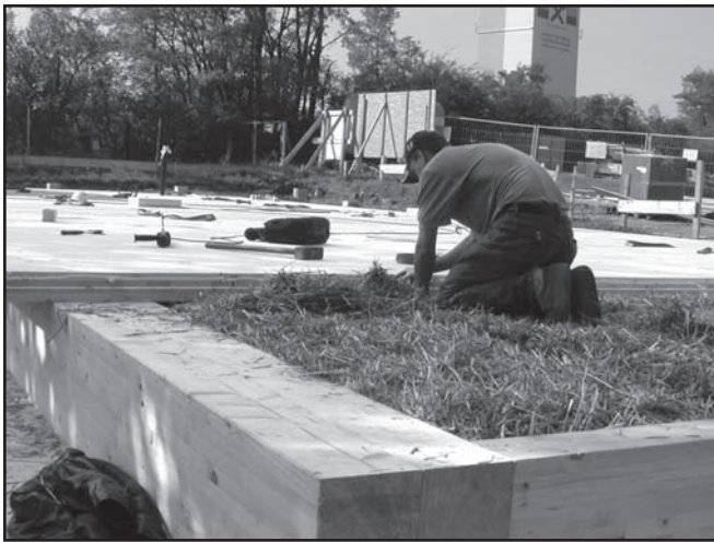
Figure 4. The floor of the S-House is insulated with a layer of straw bales sandwiched between wood panels.
