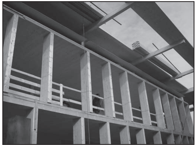
Figure 5. The roof load of the S-House’s south wall is carried by timber posts.
