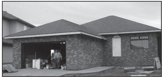
Figure 1. The Factor 9 House in Regina, Saskatchewan, has an attached garage on the north side.
