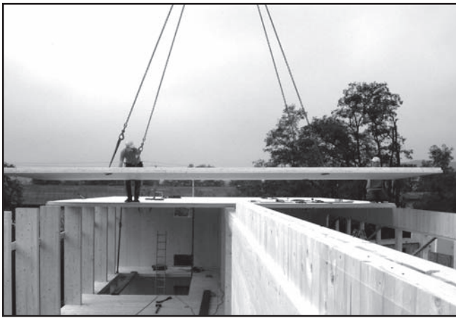
Figure 6. The S-House does not include any conventional roof framing; the structural roof consists of engineered wood panels. After these ceiling panels were set, a layer of straw bales was installed as insulation. On top of the bales, a second layer of wood roof panels was then installed by crane.
