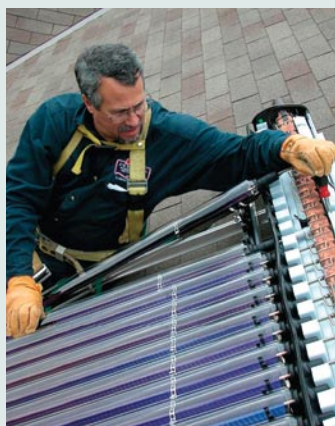
Liquid sunshine. The author assembles the Viessmann vacuum-tube solar array that produces 80% of the hot water for his home.
