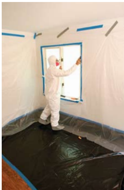
Set up a containment zone. Interior projects need a 6 ft. buffer zone that can catch dust and chips. Black plastic is a good choice on floors because chips and dust are more visible.
