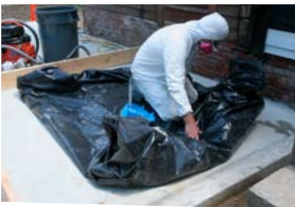
Wrap it up. When lead-removal activities are through, vacuum, mop, and wrap the floor plastic for disposal. For interior jobs, two layers of plastic are a good idea. The top layer can be the cleanup layer, and the remaining layer provides unrelated remodeling-dust-control protection.
