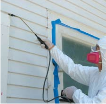
A light mist of water keeps dust down. Use a garden sprayer to mist down areas to be cut into and removed. Be careful though—wet plastic is slippery underfoot.
