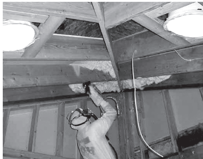
Figure 5. When Icynene is installed in a cold climate, the manufacturer recommends the installation of an interior vapor retarder. [Photo credit: Energy Smart Insulation]
