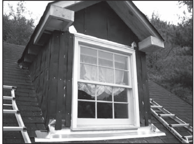
Figure 3. This photo shows vertical strips of asphalt felt installed to create a rainscreen. (Unfortunately, since the WRB in this photo is also asphalt felt, the strips are difficult to see.)
