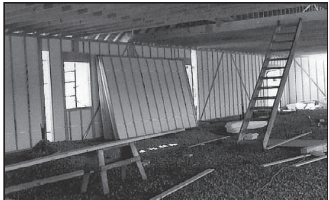
Figure 10. Load-bearing walls built with InsulWall panels require site-built headers over windows and doors.
